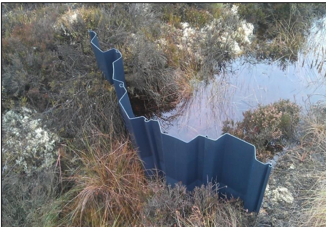
Plate 5. An example of a recycled plastic dam used to block functioning drains on a raised bog site.
